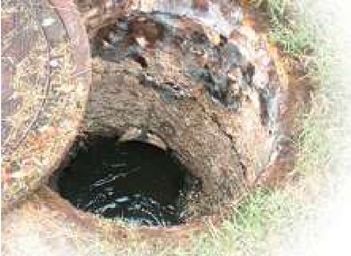
Figure 1: Corroded Concrete manhole access to a sewer line [1]
